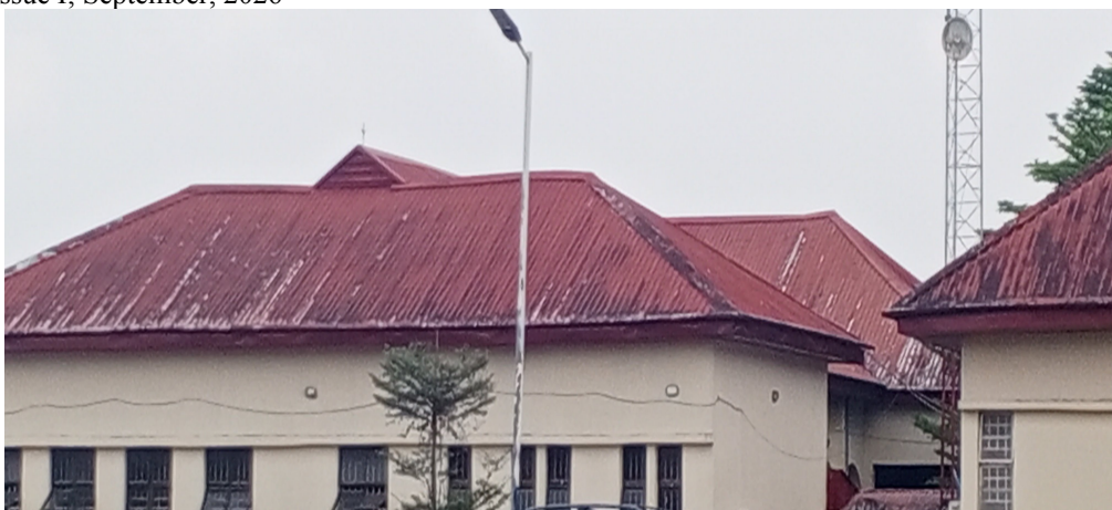
Figure 1: Severe corrosion and erosion along the runoff of aluminium roof covering at the sides against the wind direction in the Niger Delta.
